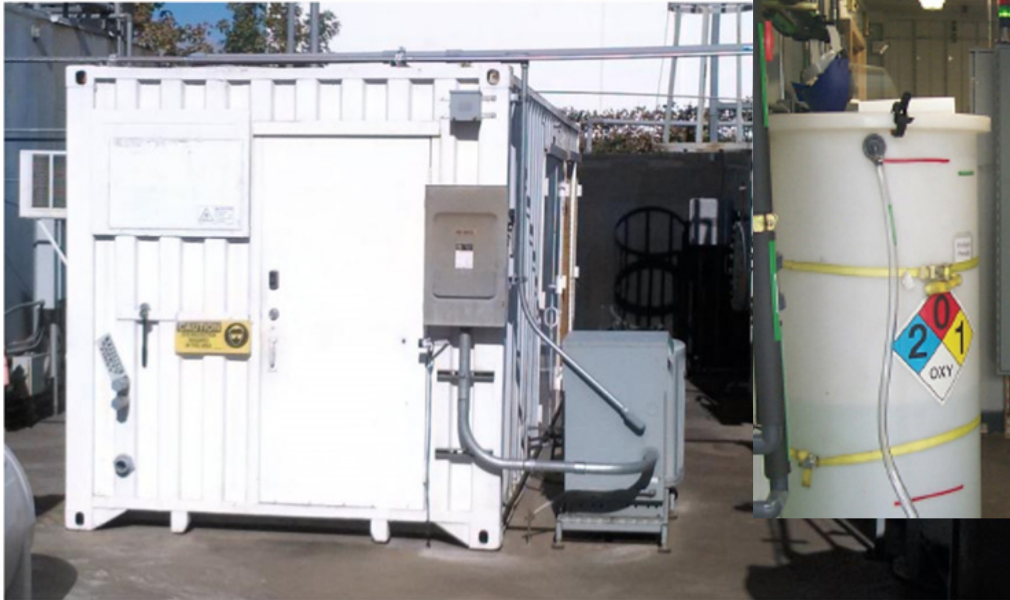
Outside view of HiPOx system
