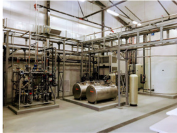
In-vessel IX Resin Regeneration System
