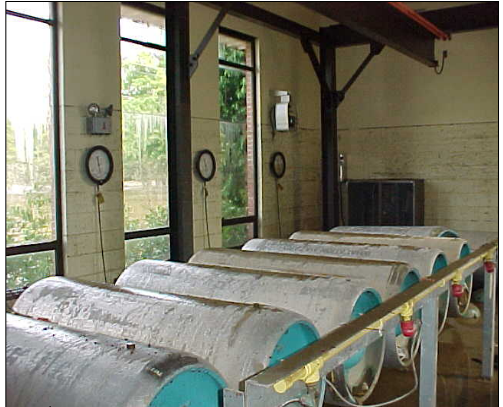
Rocky Mount, NC, water treatment plant; J. Van Hoose
