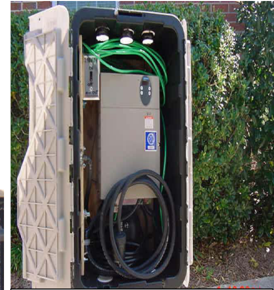
Field constructed VFD (McVay)
